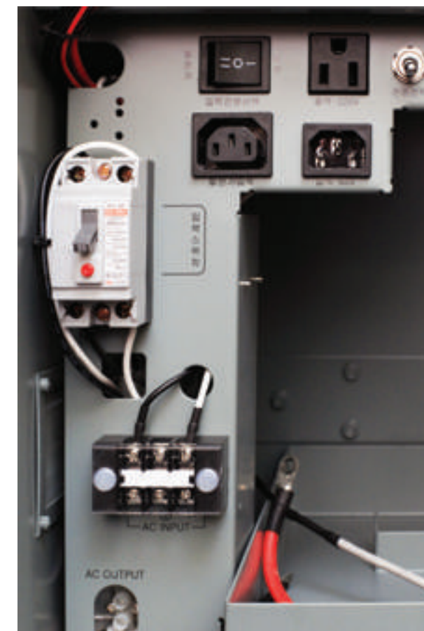
Input / Output port and circuit breaker on front side
