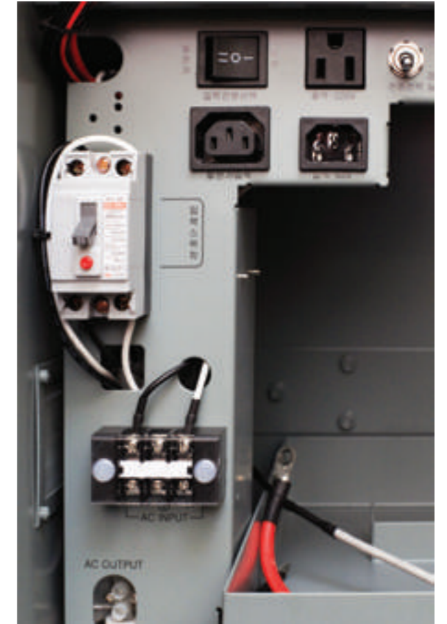
Input / Output port and circuit breaker on front side
